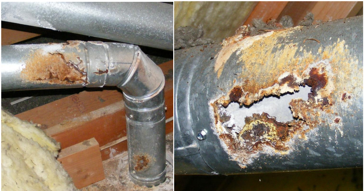
(Pictures) Severely Corroded Vent Piping
